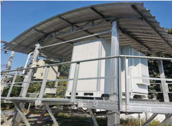
Solar Rooftop “TRUE” Chiang Rai 11 Stations
