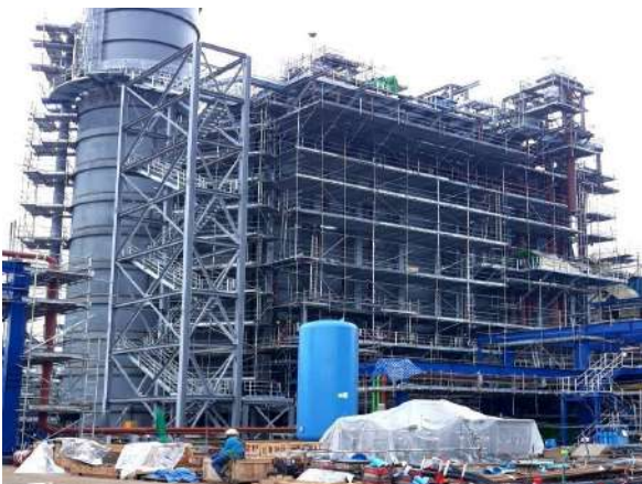
Combined Cycle Power Plant - GPSC / Sriracha Chonburi
